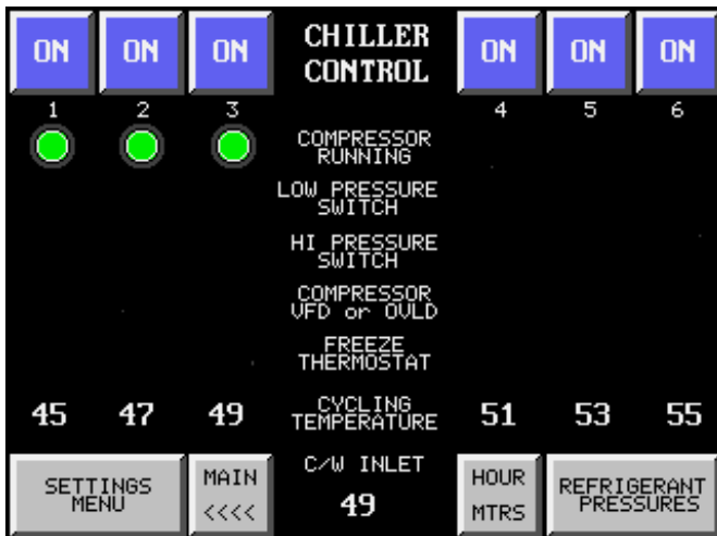
Chiller Control Screen
