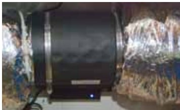
Breathe Easy In-Duct Air Purifier installed in the ductwork of the Big Oh
