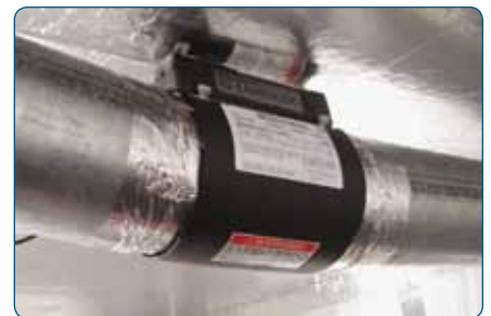
In-Duct Breathe Easy Air Purifier tube installed in the test chamber's ventilation system
